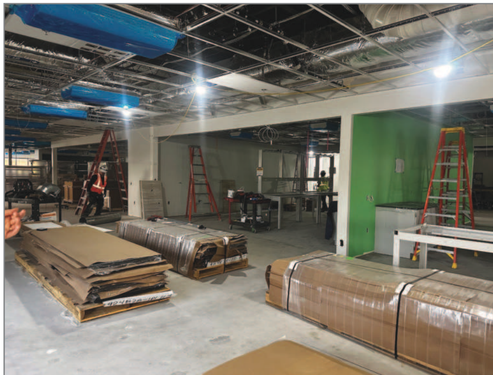
A soffit was built to house the condensate line below the level of the cabinet.
