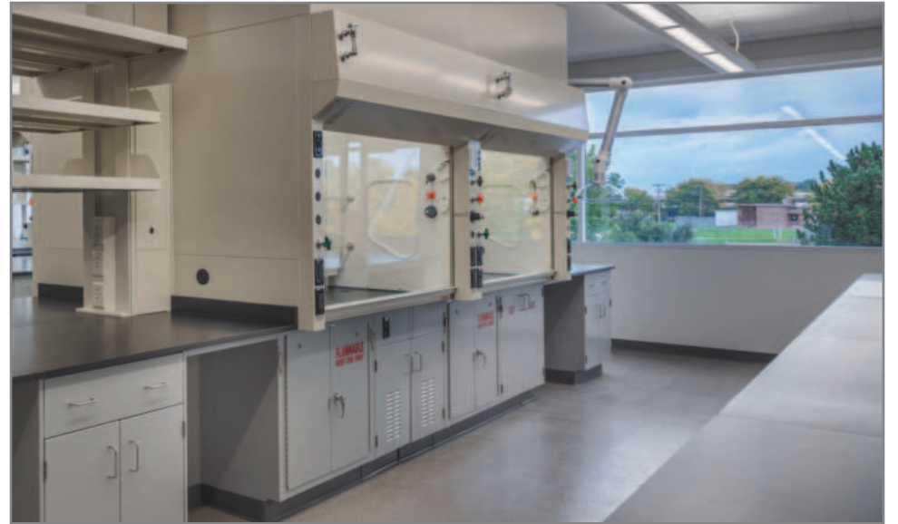
A lab at Arrowhead Pharmaceuticals in Madison, Wisconsin. The vented cabinet below the fume hood contains the lab's vacuum. Careful planning and close collaboration with architects and engineers will ensure that a lab's vacuum system is optimized for successful operations.
